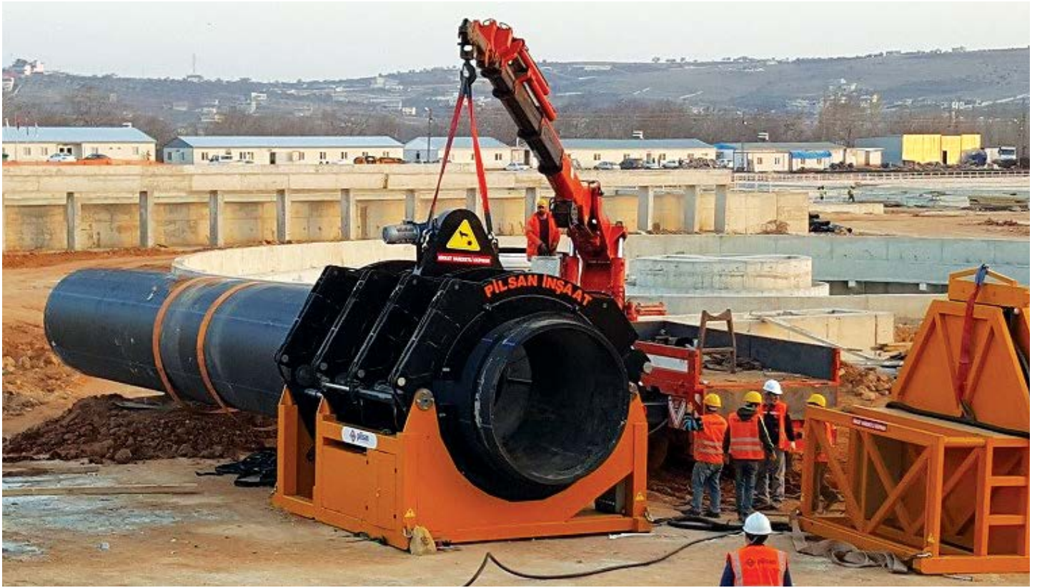
Left and right. Welding the 2000mm diameter PE100 pipeline with the Worldpoly2500 in Gaziantep, Turkey. (Courtesy of Worldpoly)
