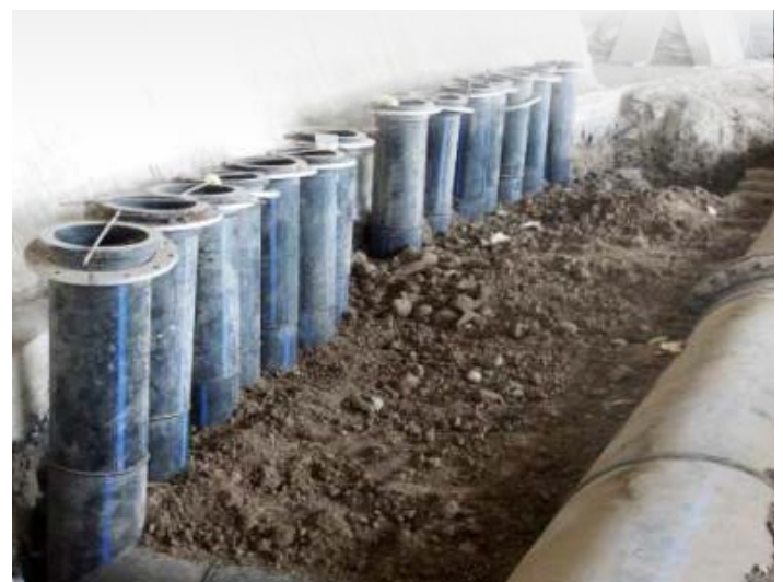
PE100 pipes installed for Central Air Conditioning system in CIDCO Exhibition Building at Vashi.
