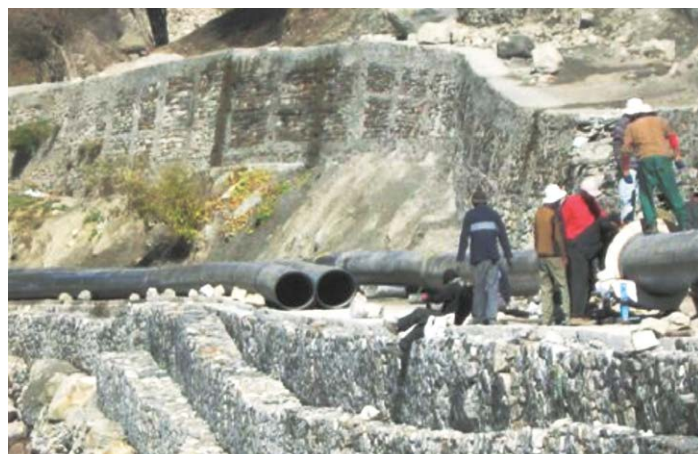
Installation of PE100 pipes for mini Hydel Power Plants in the mountains of Himachal Pradesh.
