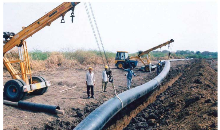
Installation of a 1000mm diameter PE pipeline for the GIDC project in Ahmedabad.
