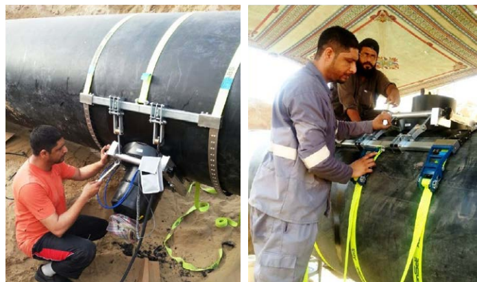
Figure 6. Electrofusion branch tees being installed for a washout and an air valve.
