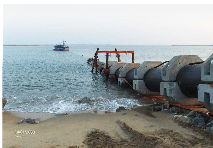
Sinking of 1600mm HDPE intake and outfall line for Minjur Desalination plant in Tamil Nadu state.
