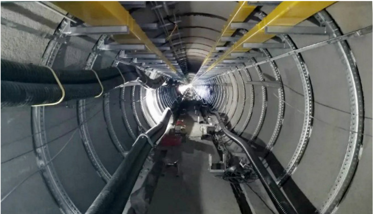
The 330kV overhead lines relocated to underground cables in Xi'an, Shaanxi. (Photo courtesy of Qingdao Hanhe Cable Co., Ltd)
